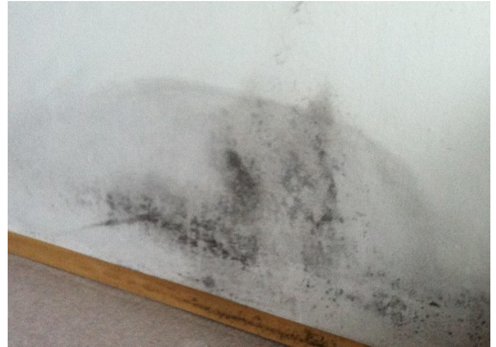
Mould behind the couch of a living room
